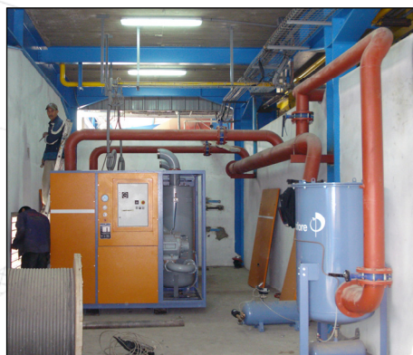
Pump room with 2 x UV30 from 2010
